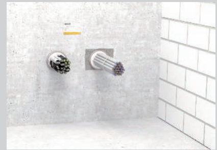
Pipe shells with full assignment with cable bundles and electrical installation pipes.
