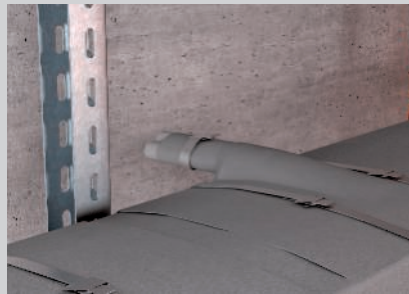
Cable exit with bandaging.
